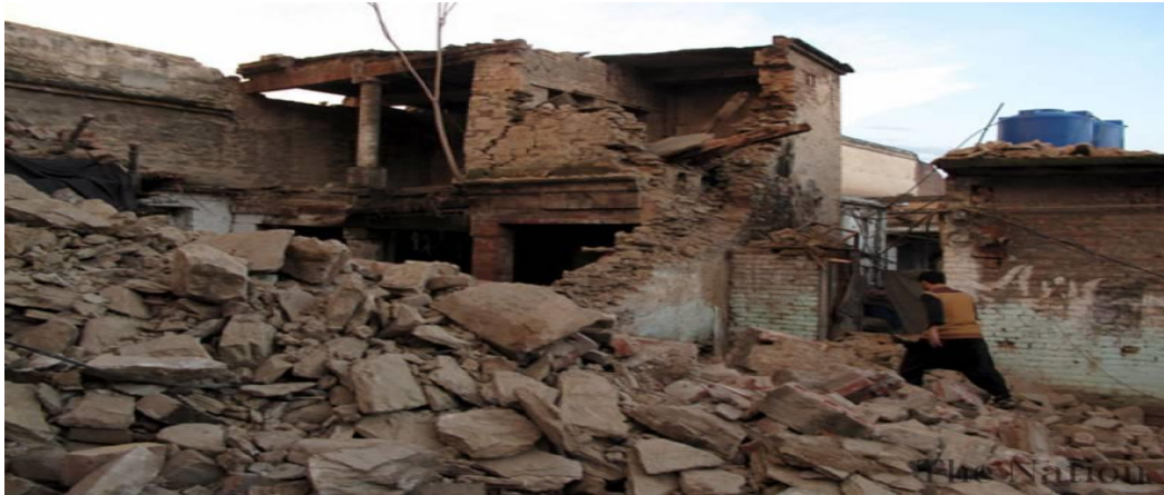
Houses destroyed in Oct 26, 2015 Earthquake in Northern Areas of Pakistan 3 .
